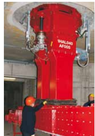
BAS 3, integrated in concrete silo
